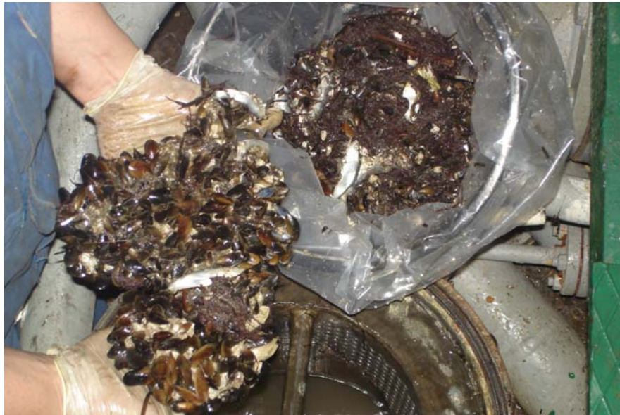
Figure 1: Clogged sea chest
