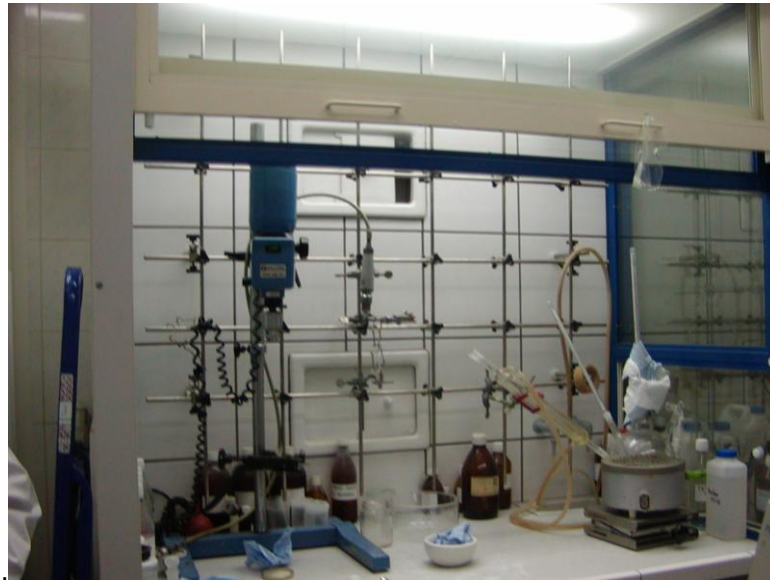
Figure 1: Ventilation system: LEV
