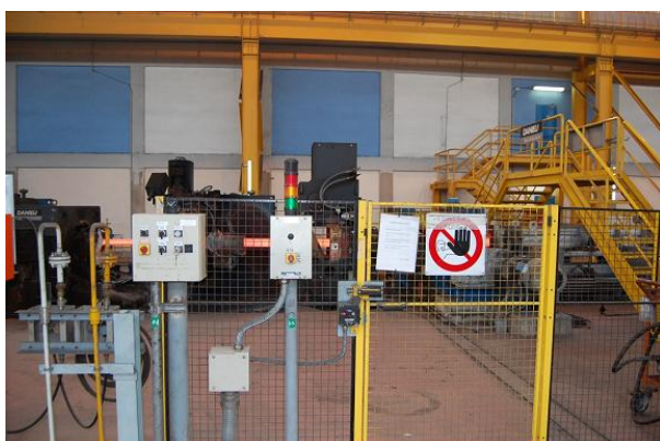
Figure 4. Access and exit control system
