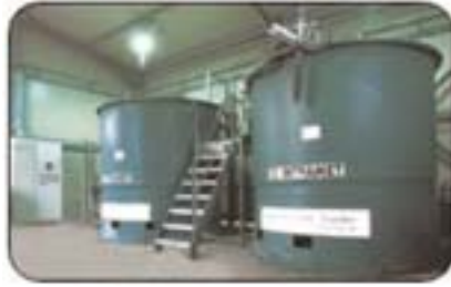
The biological degreasing system
