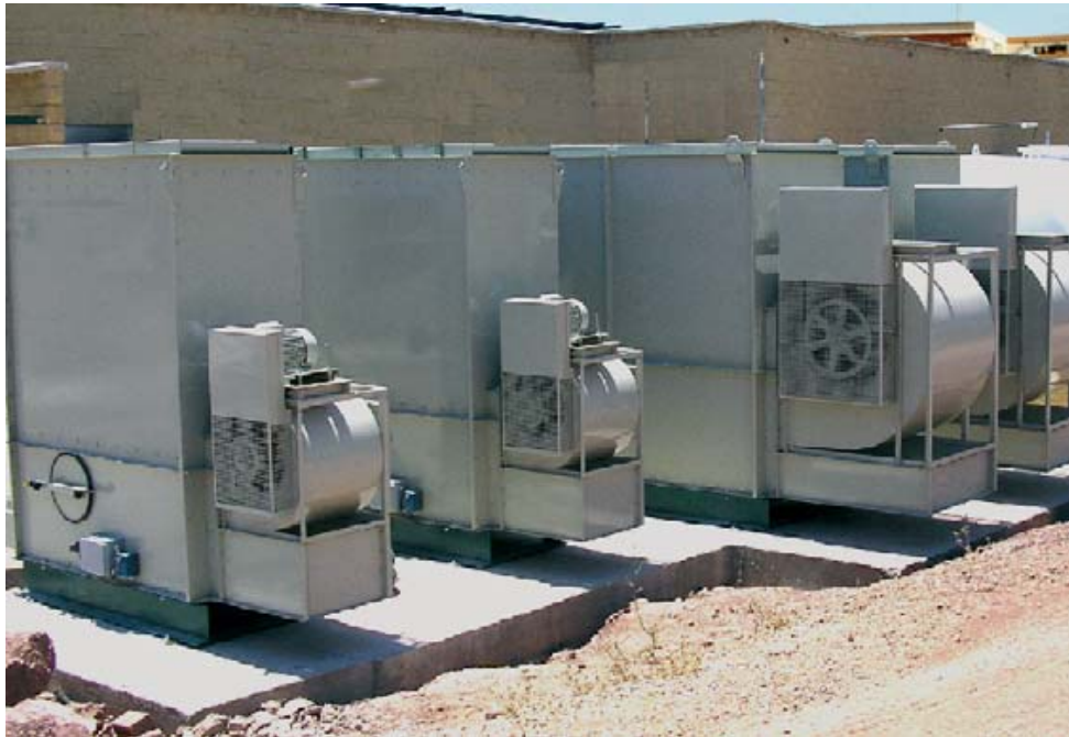
Picture 2: Cooling towers
