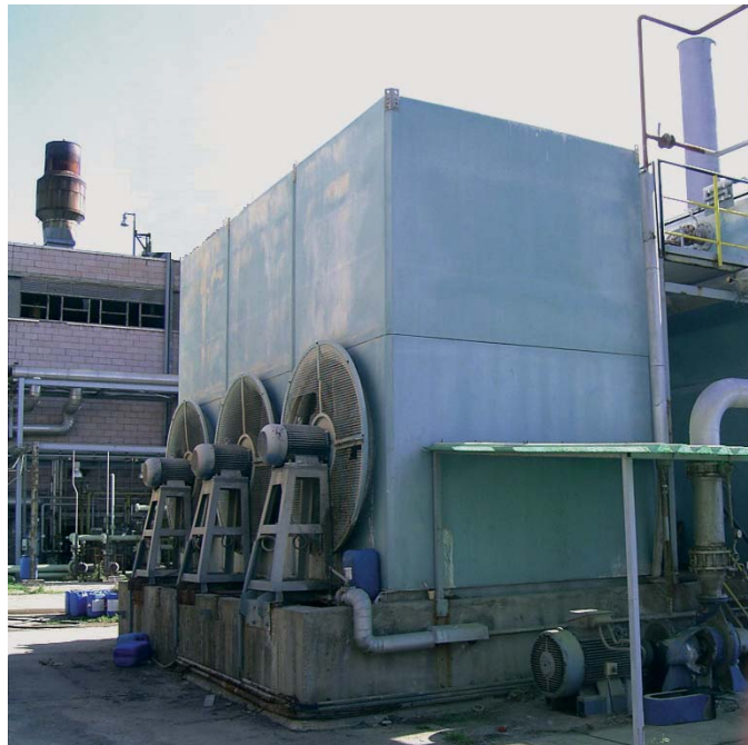
Picture 3: Cooling towers
