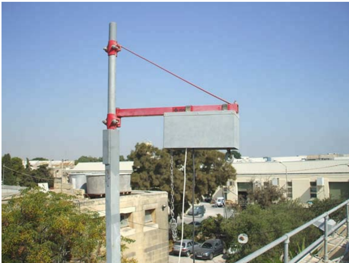
Fig.6 Hoist device located on roof area to assist technicians in transporting the pharmaceutical process waste bags
