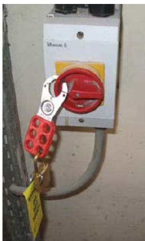
Fig. 9 Electrical Isolator Locked off and tagged
