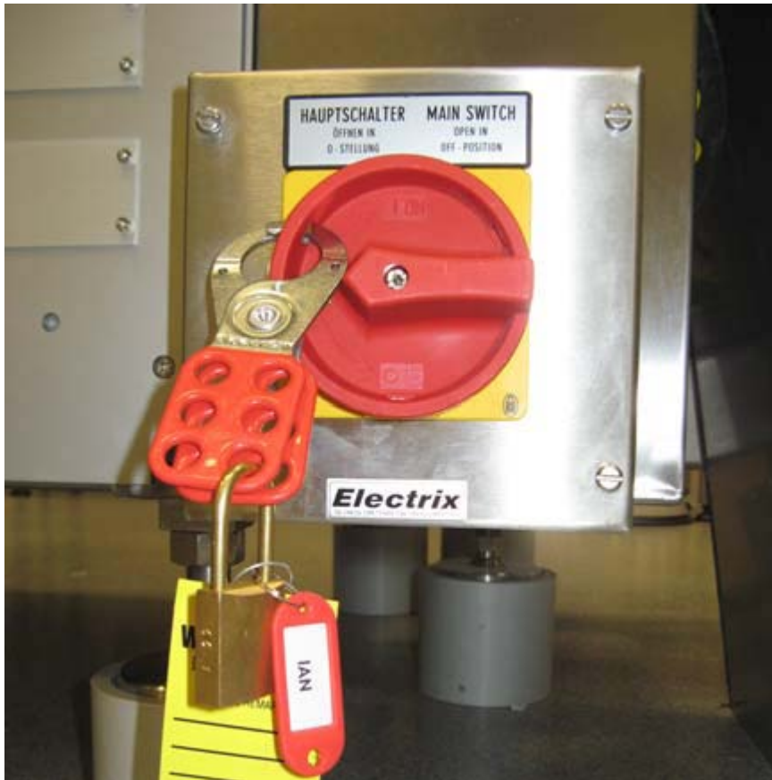
Fig.7 Lock off device used to isolate equipment prior to a maintenance activity
