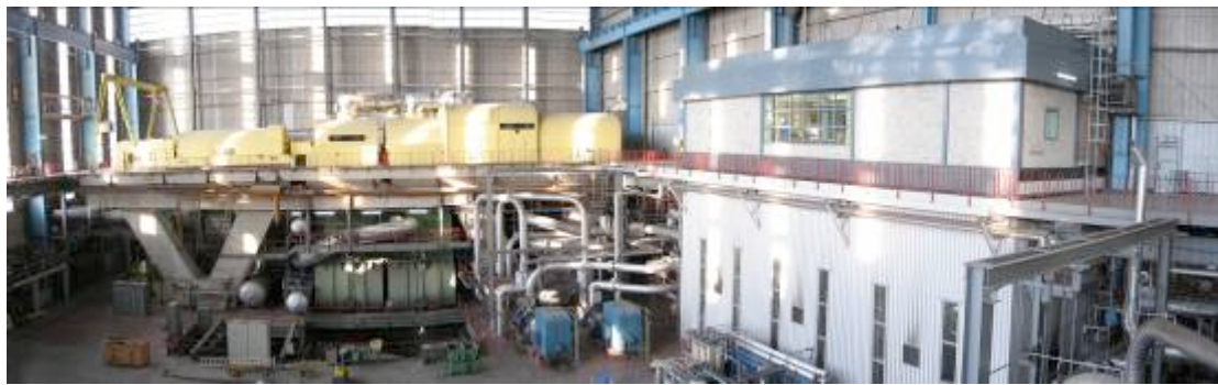
Figure 1: Steam turbine and machine room at the thermal power station of Langerlo
