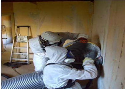
Removal wallpaper and plaster with concrete grinder with direct extraction, additional exhaust ventilation of the working area.
