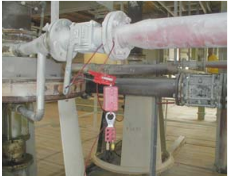
Lockout on a pipe to prevent unintentional release of hot stem. The master lock in the red box blocks the clip. The master lock cannot be removed before the two workers have removed their personal keys
