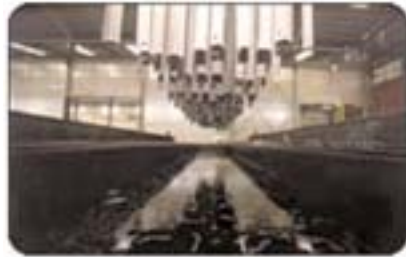
The activated pickling system
